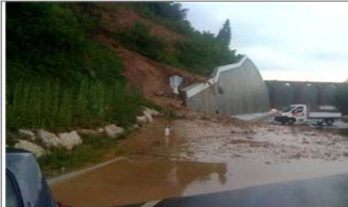
mudslide along slope protection (Varese 2009) - courtesy of Varese news (photo by Pierangelo Scotti)
