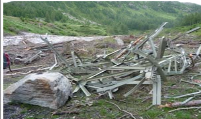
destroyed high-voltage line hit by a snow avalanche (Zwischbergen valley, Switzerland) - photo by Stefan Scheer (JRC)
