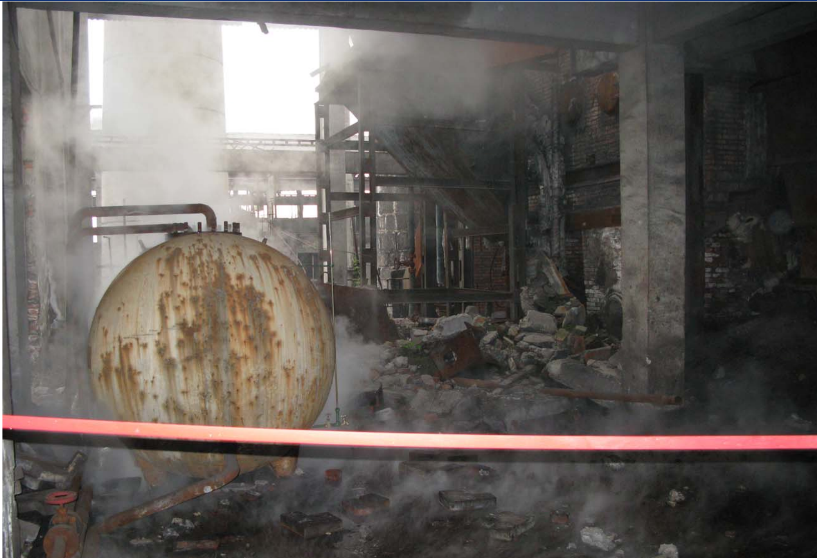
Damage to production building
