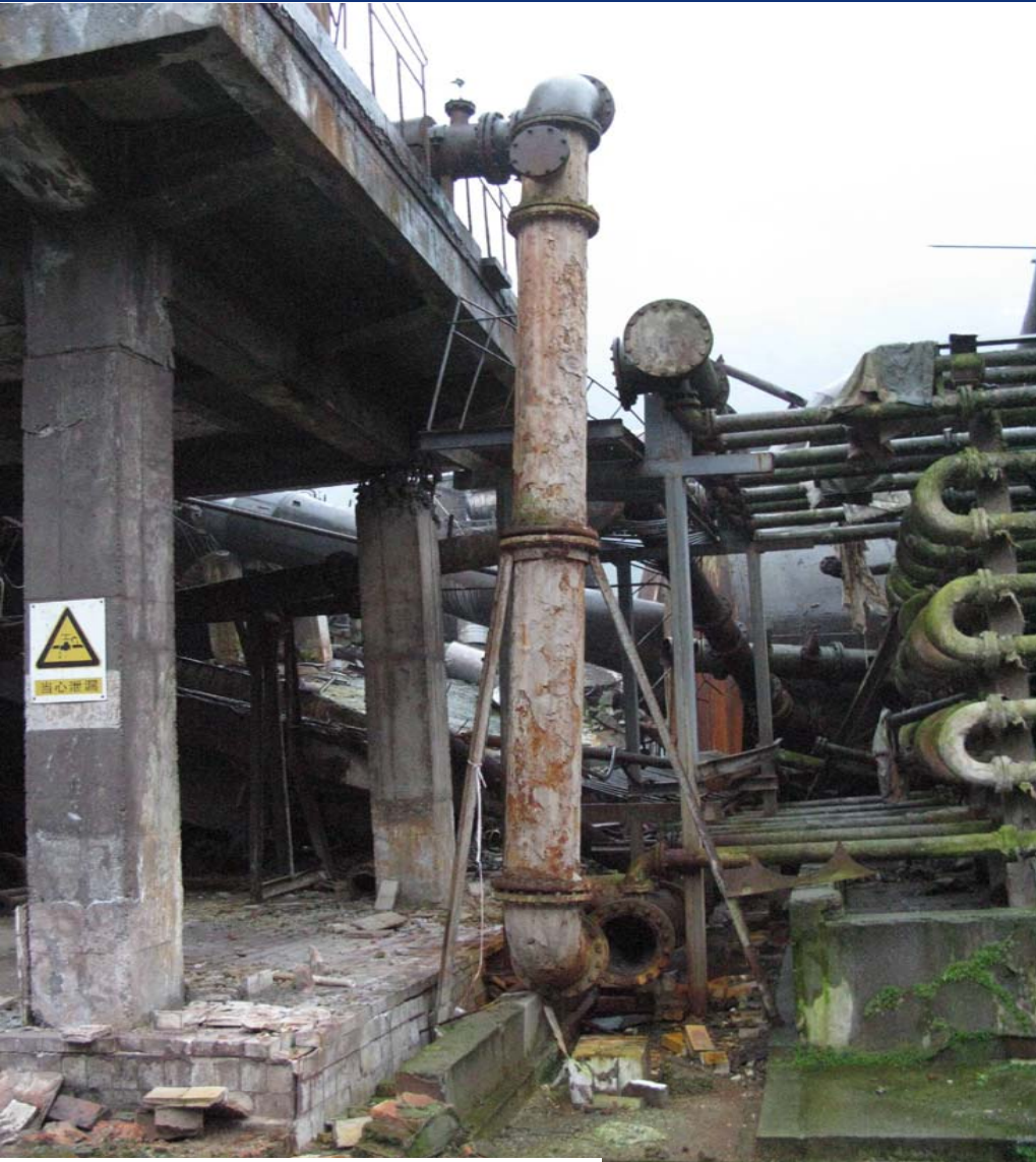
Pipe connection failure
