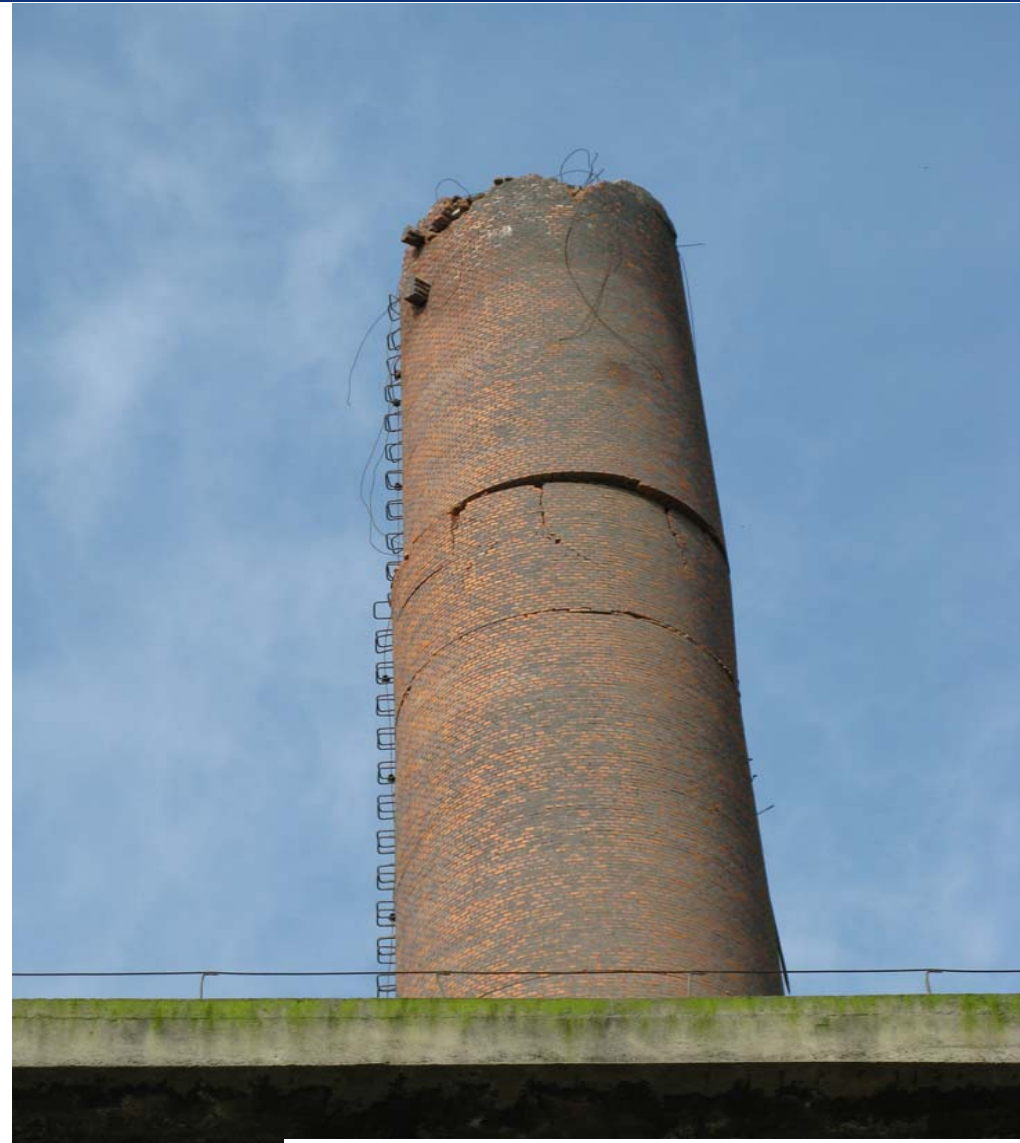
Damage to masonry chimney
